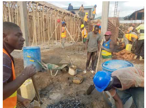
The construction of the refectory is diligently continuing in Gisenyi. The premises under the refectory, library room and computer room are very strong.
